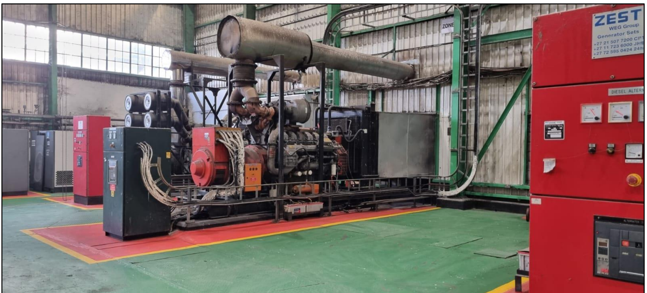
FIGURE 1.2: EXISTING POWERHOUSE WHERE NEW 17MW TA IS PROPOSED (ONE 3.5MW TA WILL BE REMOVED)
